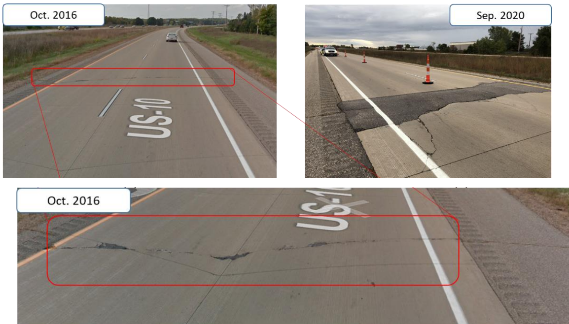
Figure 13. Google Earth® images of U.S. 10 in Portage county (site # 1) prior to buckling showing spalls, shoulder cracking, and asphalt patching (left and bottom). Image on the right, collected during the September 2020 field survey shows the same location patched with full-depth asphalt following the blowup.
