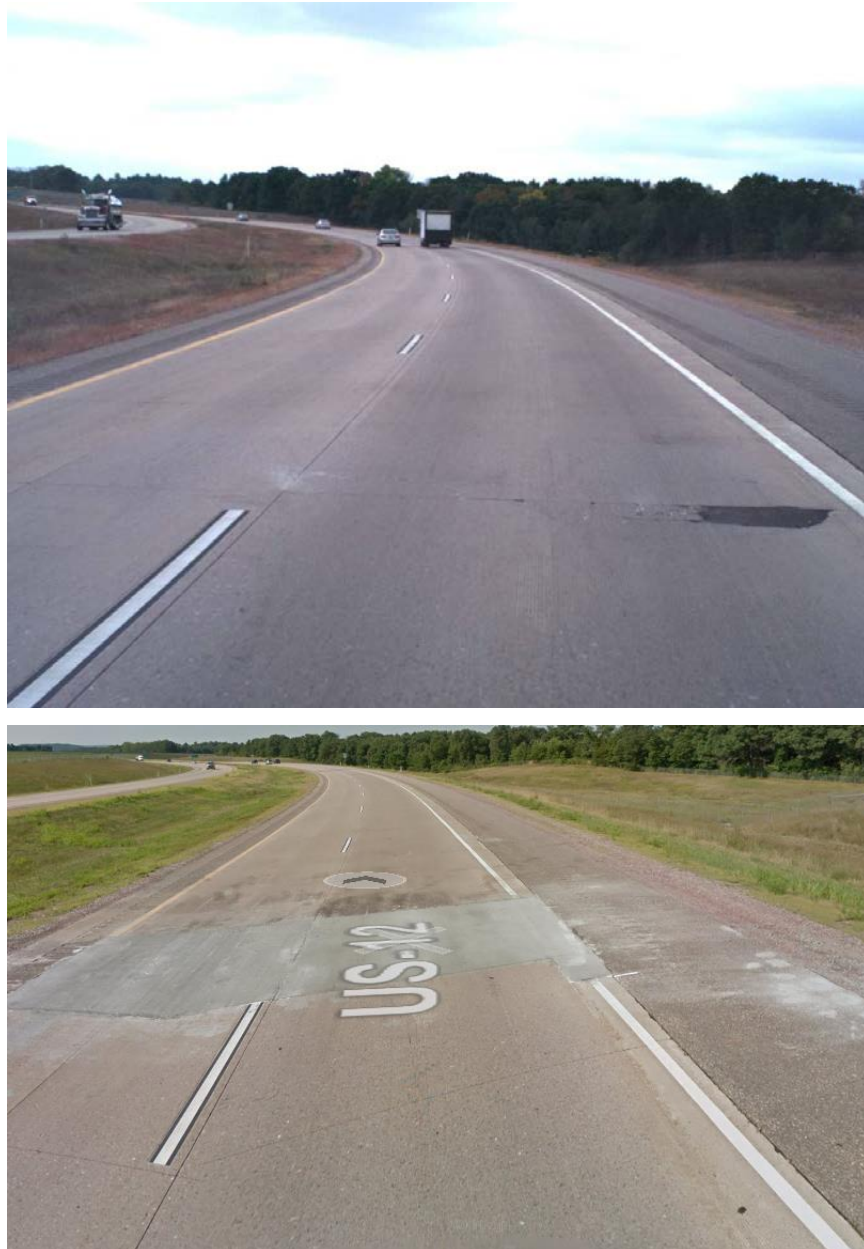
Figure 14. October 2017 Google Earth® images of U.S. 12 prior to buckling showing spalls and asphalt patching (top). July 2018 Google Earth® image of the same joint following buckling (bottom).
