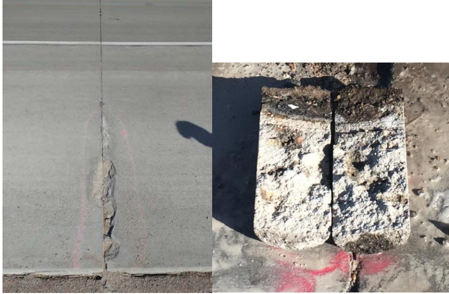
Figure 43. Spalling along the shoulder joint where incompressibles infiltrated after only 1.5-years of service on I-80 in Nebraska (left). Core taken in the spall area (right).
