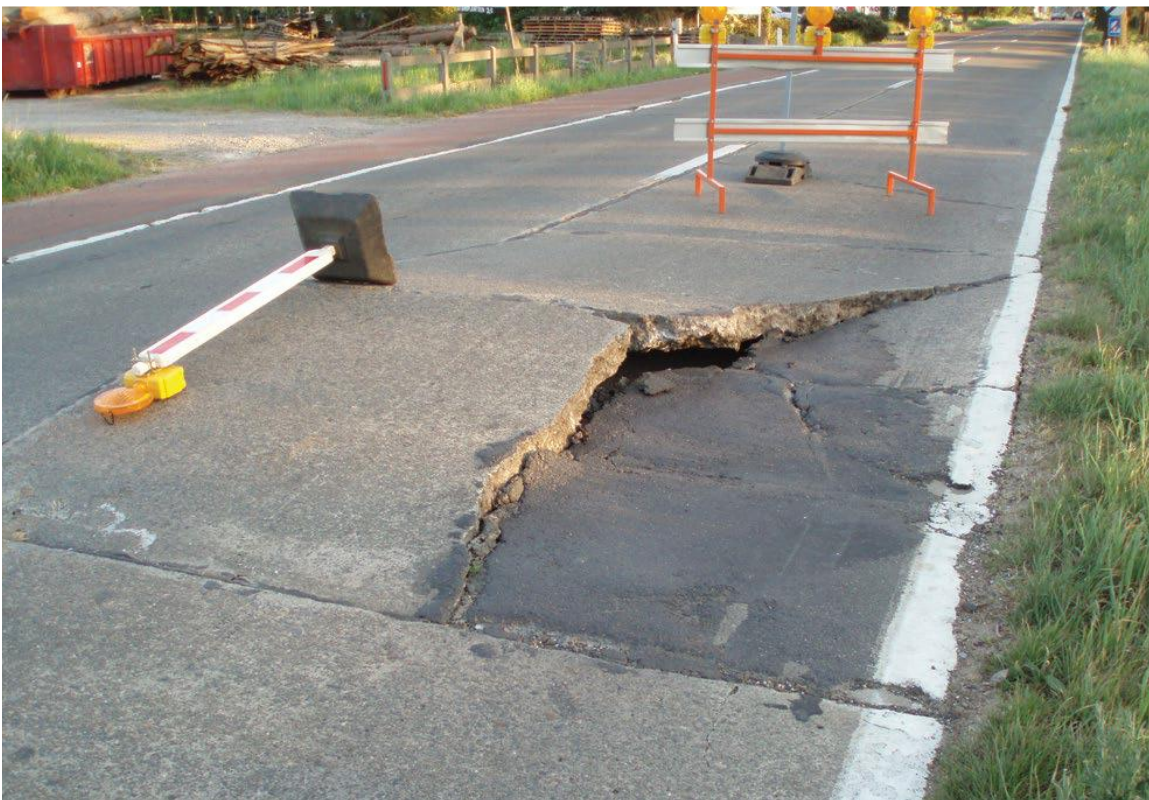
Figure 45. Buckling caused by HMA patching (Rens 2018).
