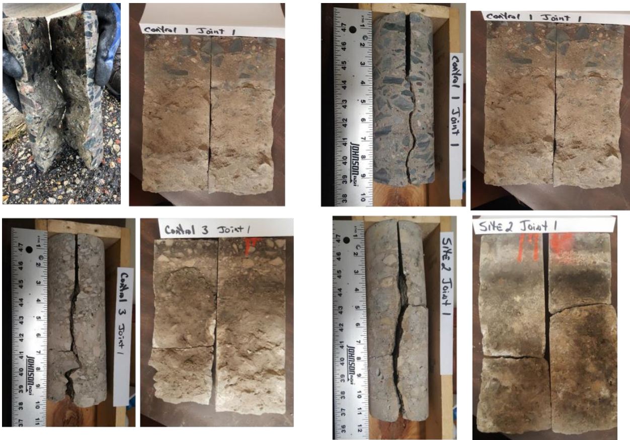
Figure 16. Cores from control sites taken from transverse joints and core holes showing no spalls in the lower portion of the joint.
