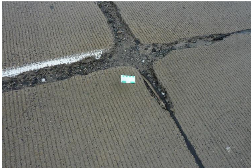
Figure 65. Deteriorated Joints on Highway 417 (Chan et al. 2020).
