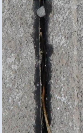
Figure 8 Unsatisfactory Filled Joint
