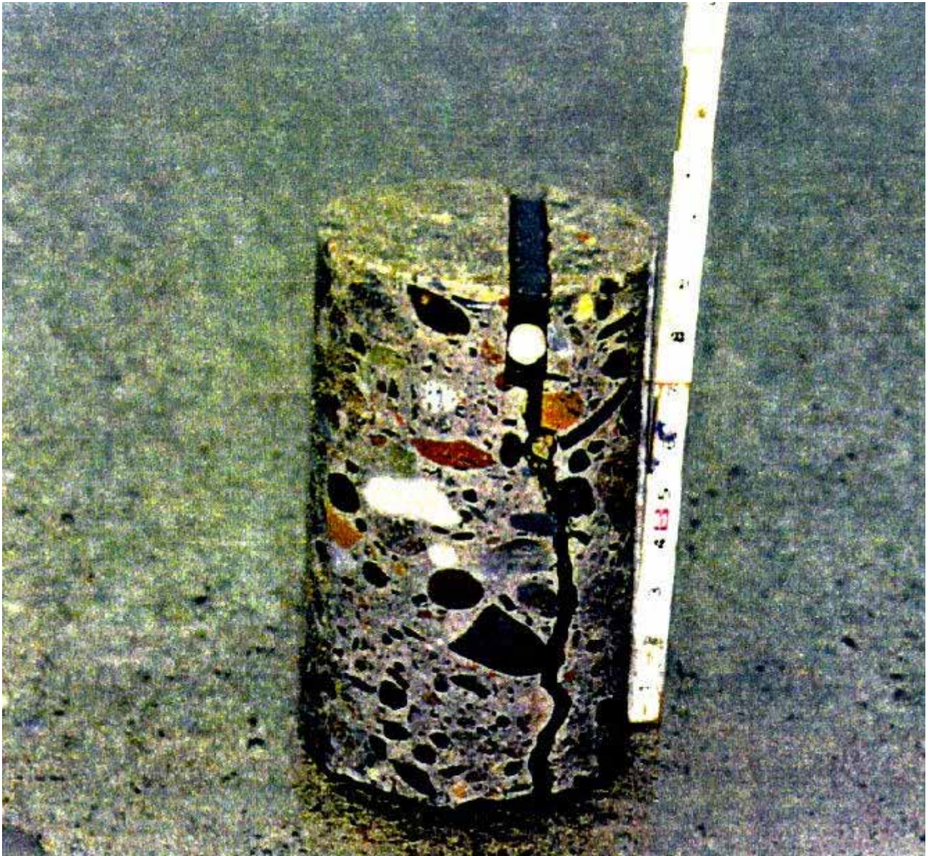
Print 3. Core of sealed joint at 21 years of age -- six meter joint spacing. No distress.
