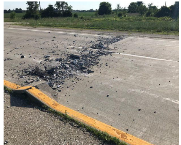
Blowup on Hwy 14 in Rock County
