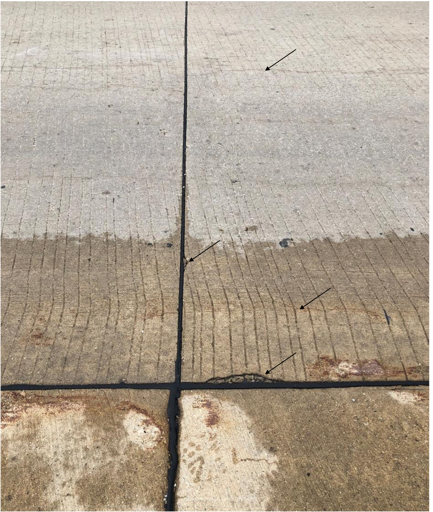
Figure 1-3 Crack in Pavement, Spall at Curb, Spall in Transverse Joint where Tining Crosses, Note also cohesive failure in hot pour- This sealant would have been rated as 0% missing
