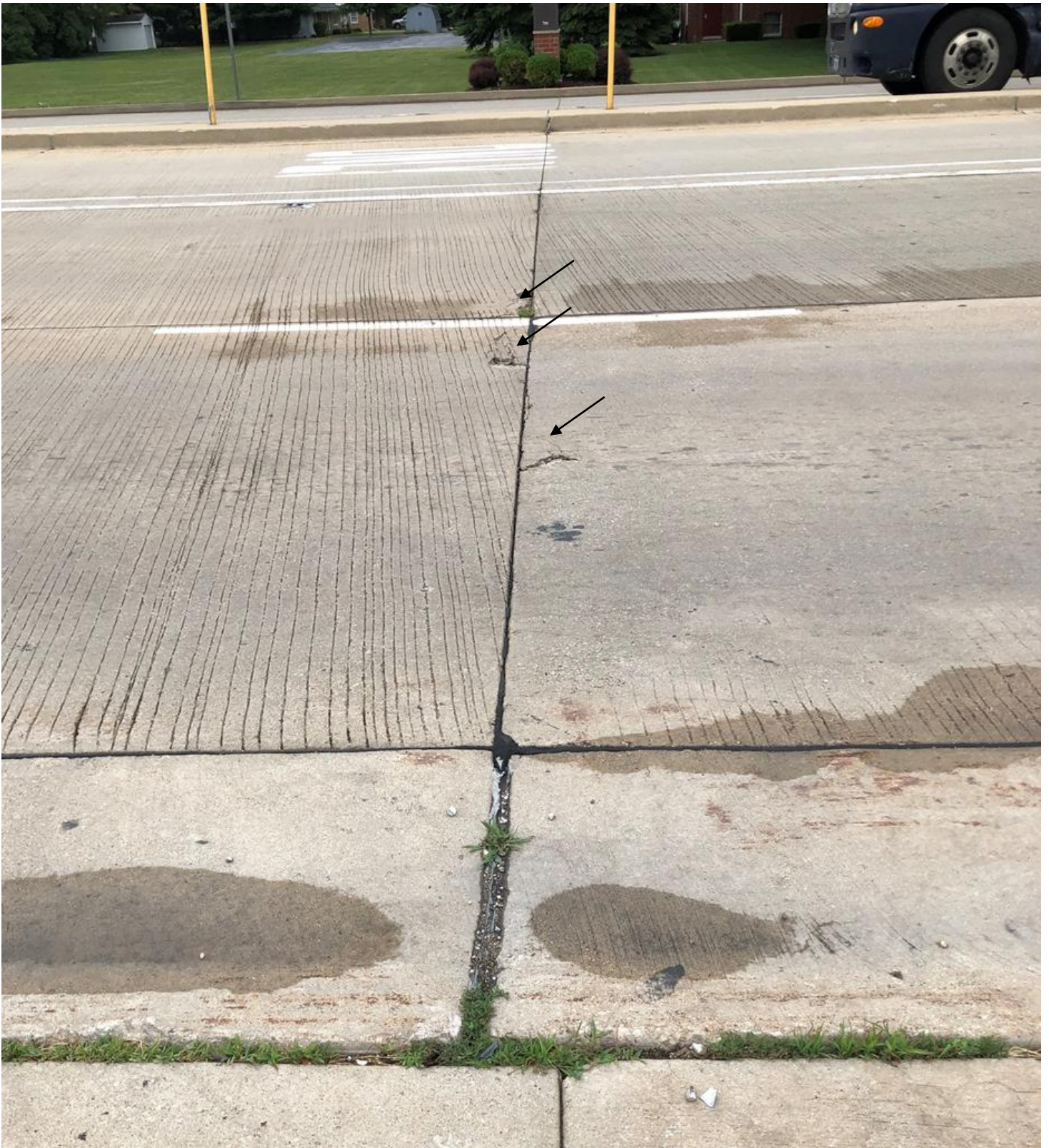
Figure 1-4 Note Delamination Occurring and Lack of Tining on Right Side of Joint
