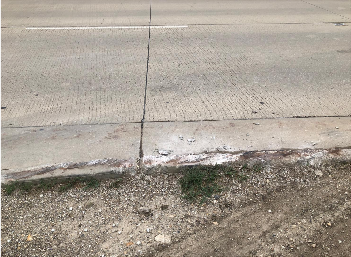
Figure 1-6 Curb Damage and Construction Debris at Approximately 3232+00
