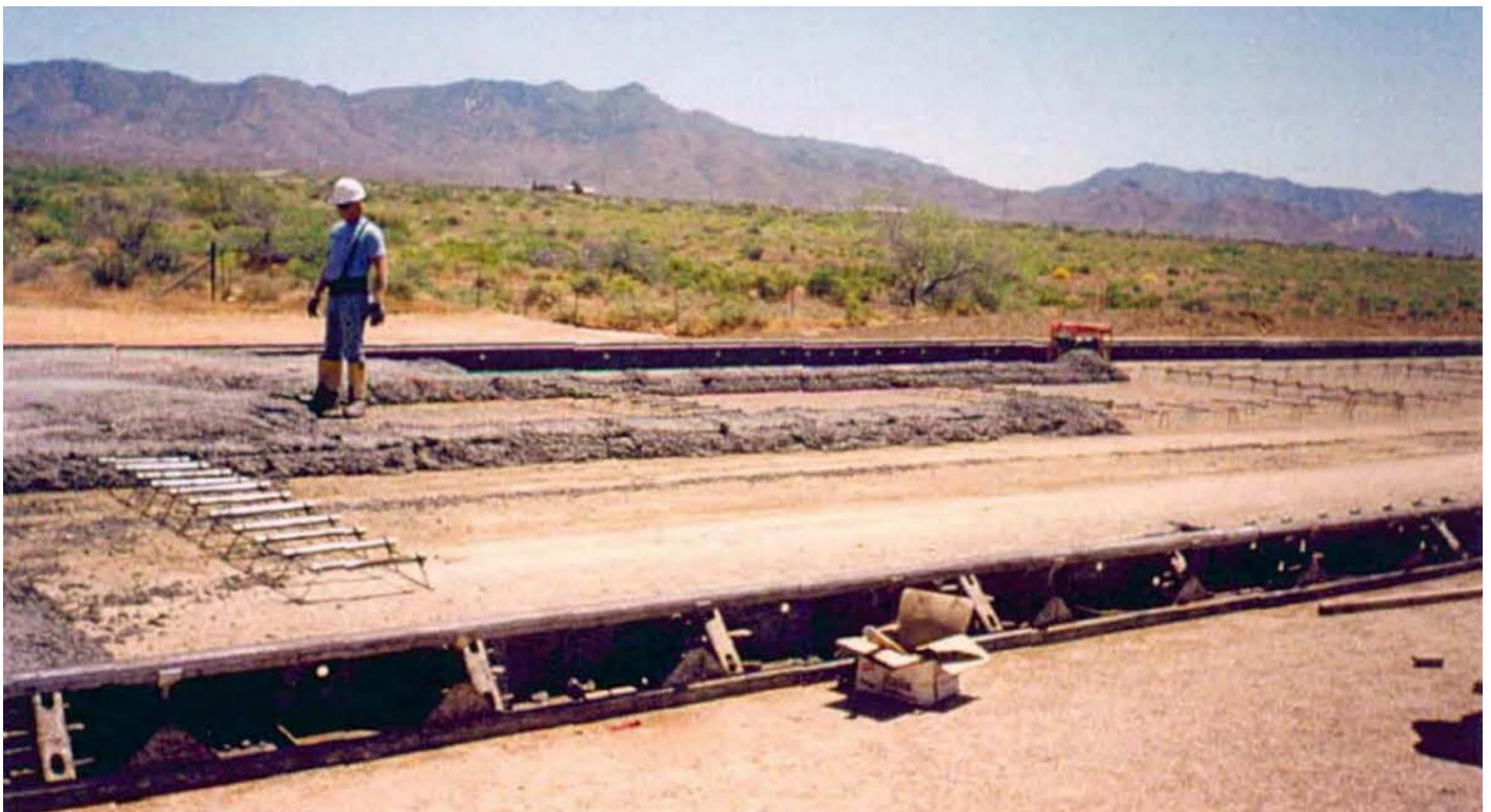
Figure 3-2 Indicates Dowel Baskets and Tie Bar Stands and Concrete Spotting to Hold Them in Place
