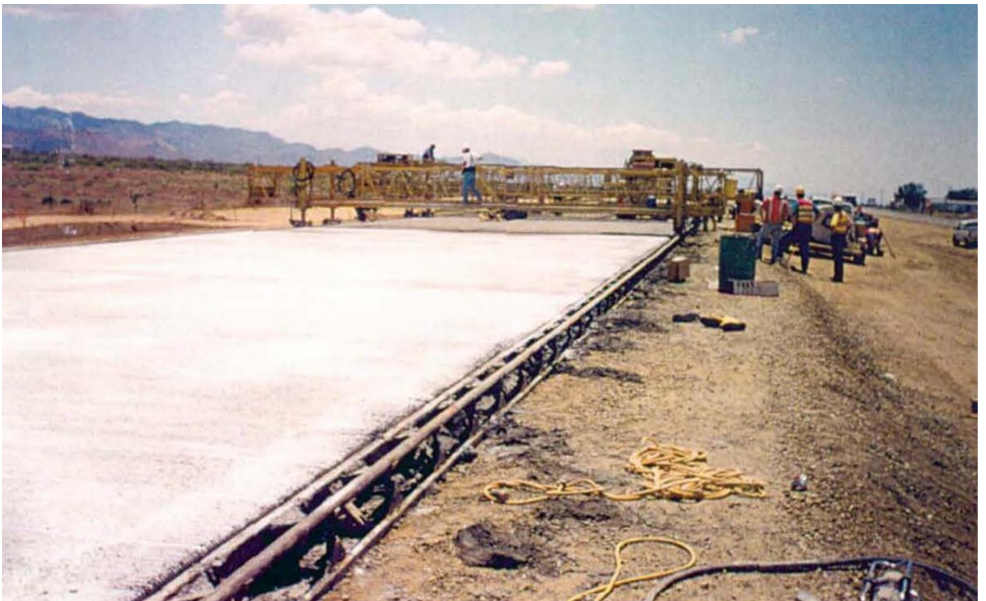
Figure 3-4 Photo of Inadequate Coverage of Hand Sprayed Curing Compound
